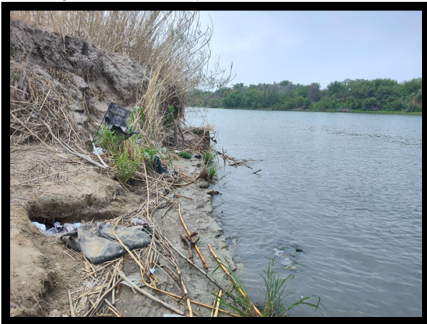
Close-up view of sheer, eroding banks on U.S. side of river (Note strata of exposed claypan.)
